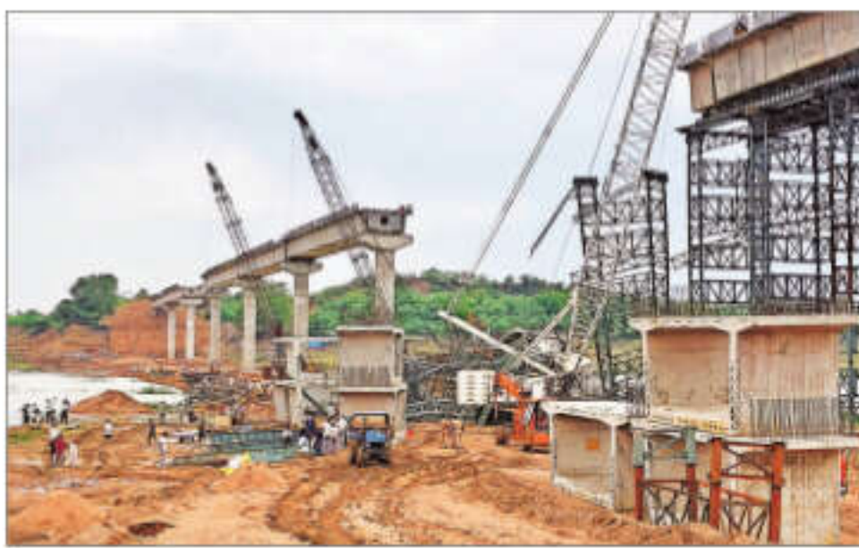
The site of Hamirpur bridge collapse on Friday. PTI
